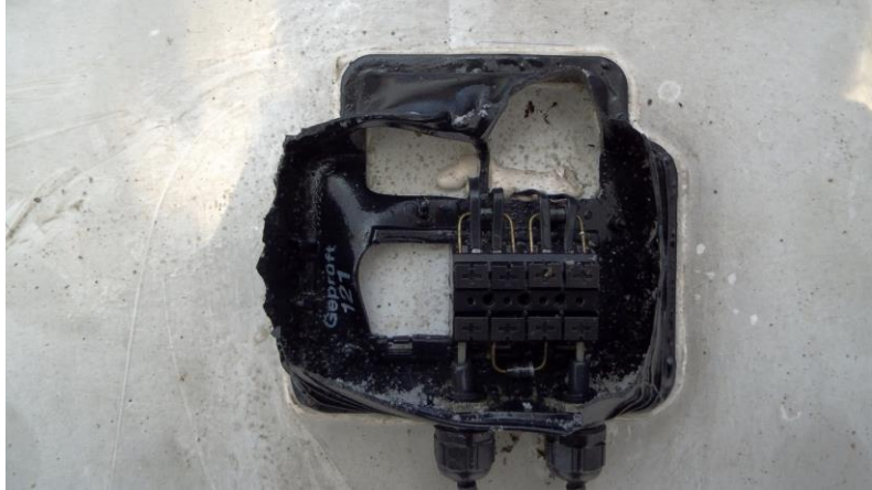
Burned and damaged junction box
