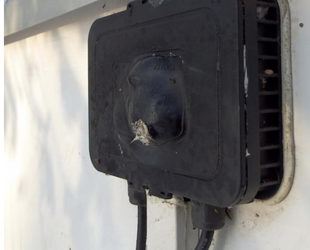
Bloated junction box
