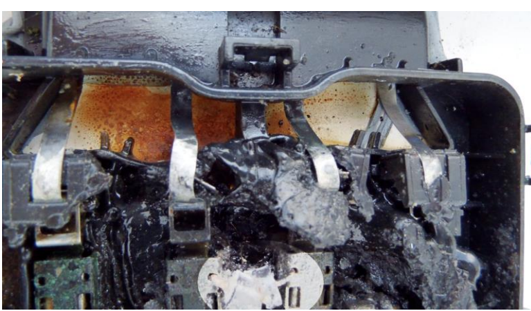
Burned diodes and junction box
